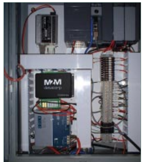
Figure 2: Typical PLC panel assembly with a "push" Internet gateway device.
